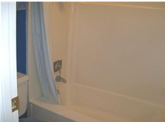
Tub is self contained unit.
