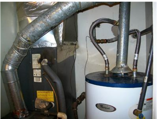
Storage Closet in Hallway contains Hot Water Heater and Furnace for convenience and ease - NO crawling under the house to change filters in this home!
